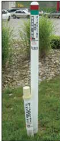
2. Linemarker and cathodic protection test station
